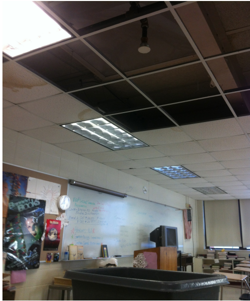
Figure 3. Rain inside the traditional classroom space Spring 2013
