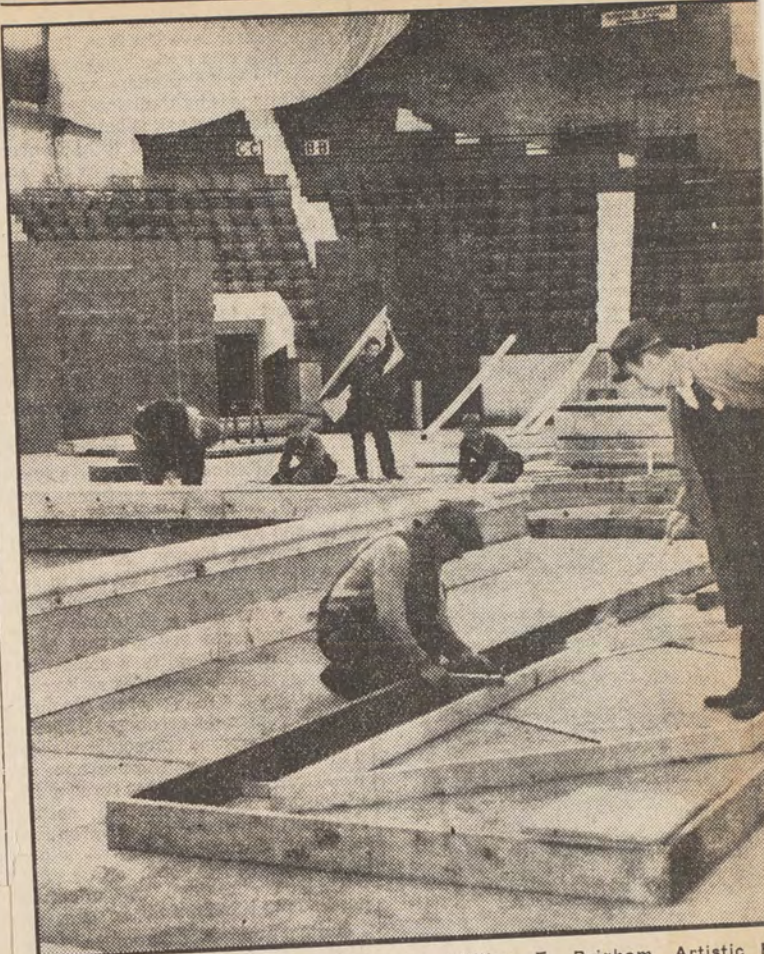
This View of Huge Arena, Showing William E. Brigham, Artistic Director in Foreground, Gives a Glimpse of Features of the Exhibition Opening in May. Mr. Brigham is Superintending the Construction of Frames for the Pool, a Corner of Which Will Surround the Pool for Aquatic Plants, a Corner of Which is Shown on the Left Can Be Seen a Portion of the 12-Foot Fence Which Will Enclose the Pool and Be Made to Resemble a Stone Wall. The Motif of This Year's Show by the Associated Garden Clubs of Rhode Island, is a Formal Italian Garden. The Pool, and a Cascade at the East End of the Hall Are to Be Featured in the Show Will Continue Through Next Sunday.
