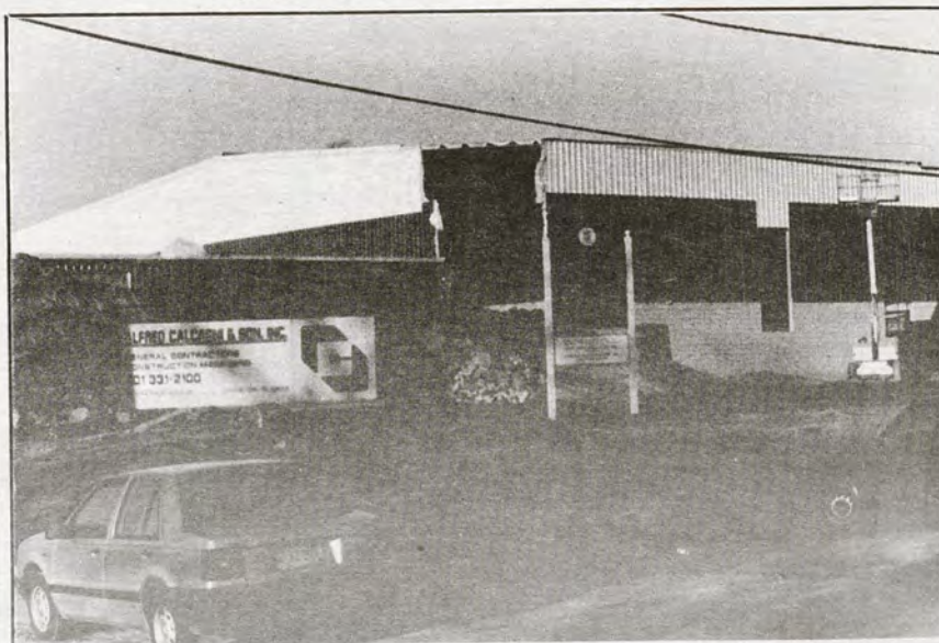
Construction on the RIC Rec Center, stalled repeatedly from the beginning, will be taken over by Holiday Health, Inc. Construction will resume in time to open the center by Fall. -Anchor photo
