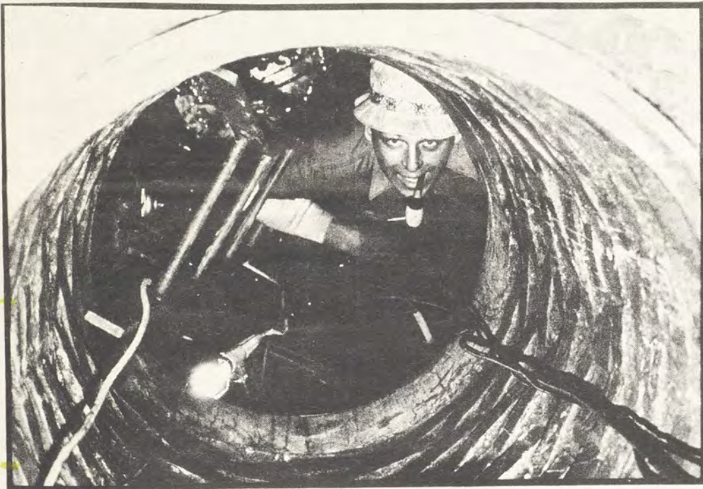
Maintenance Worker peers upward while working to restore power to the dormitories during recent 45 hr. power outage. Photo by Dave Zapatka.
