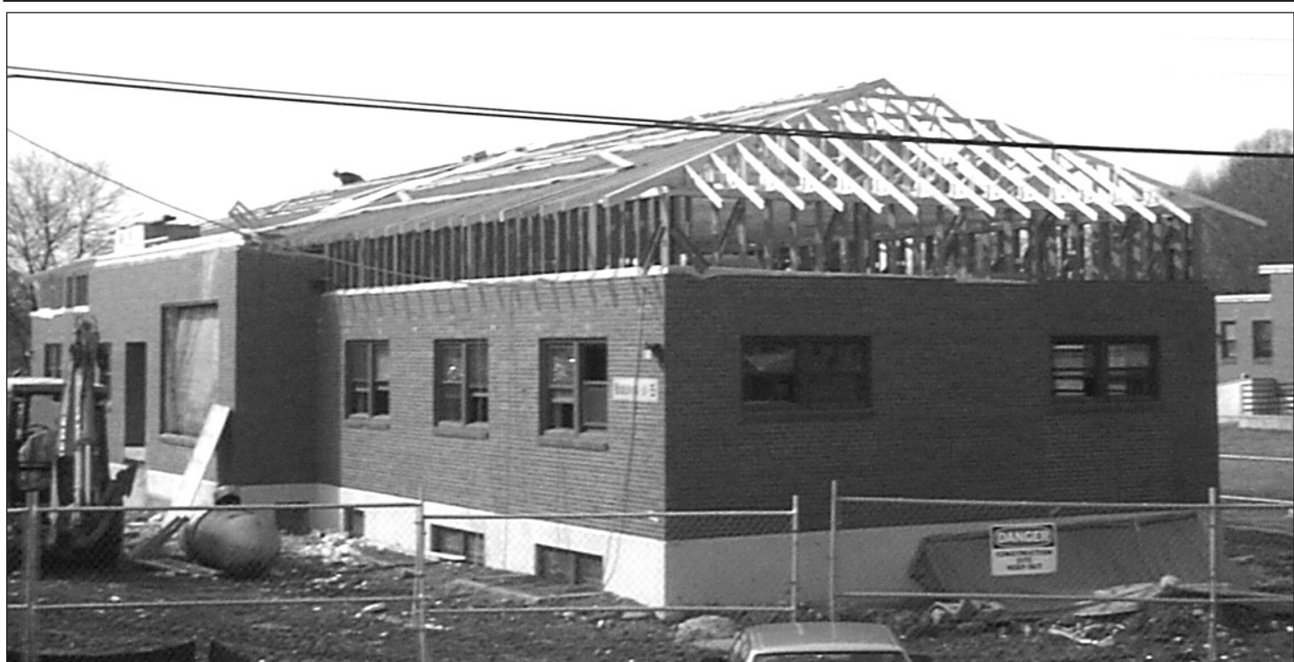
RAISING THE ROOF: Building 5, above, and the neighboring Building 4, two of the former Department of Children, Youth and Families buildings being renovated for use by Rhode Island College, is getting a new hip roof with architectural shingles to go with the extensive interior renovations. The old flat roofs, which were in disrepair and prone to leaking, are being replaced with the more aesthetically-pleasing hip roofs. The renovations, which will provide a new home for the Bursar and Records Office in Building 4 and for purchasing, payroll and accounting in Building 5, are expected to be completed in early fall. (What's News Photo by Gordon E. Rowley)
