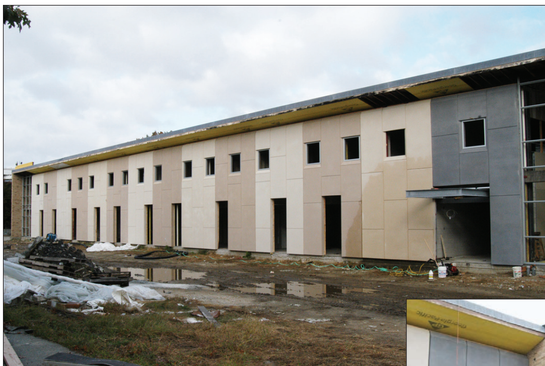
NEW LOOK: Workmen recently installed the new siding on Alger Hall, soon to be the new site of the School of Management and Technology. Sections of the new siding, a composite of concrete and Fiberglas, were prefabricated in Central Falls and installed at the rate of three a day.
