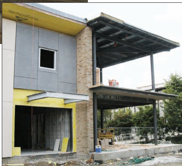
Pictured at right is an exterior view of the southern end of Alger Hall where the student lounges will be located.
