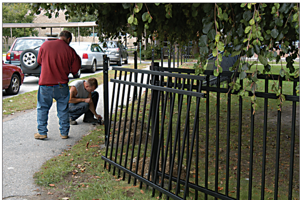
BARNARD FENCE: A crew from New England Fence installs a wrought iron fence at the Henry Barnard School as part of the ongoing Special Capital Project. Framing the original HBS entablature from the 1928 Hays Street site (top photo), sections of the fence may be purchased in honor or in memory of a loved one with an appropriate plaque installed to recognize your gift. For further information, contact Patricia Nolin at 401-456-9854 or pnolin@ric.edu .
