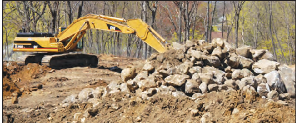
BEFORE: Construction has begun on the new residence hall on Sixth Avenue.
