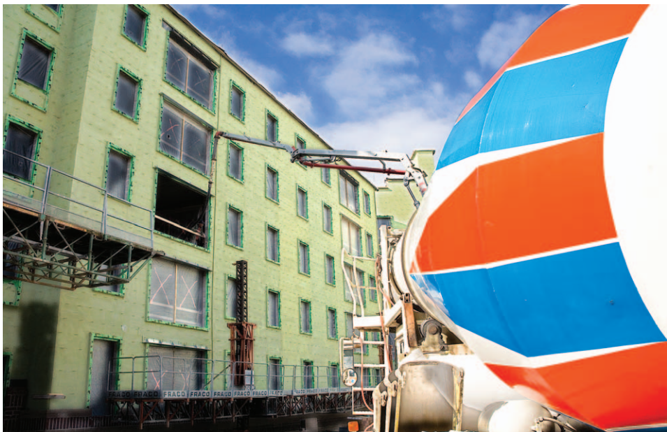
THE SKYLINE IS CHANGING: Cement trucks continue to pour into the construction site as the new residence hall towers over the RIC campus.
