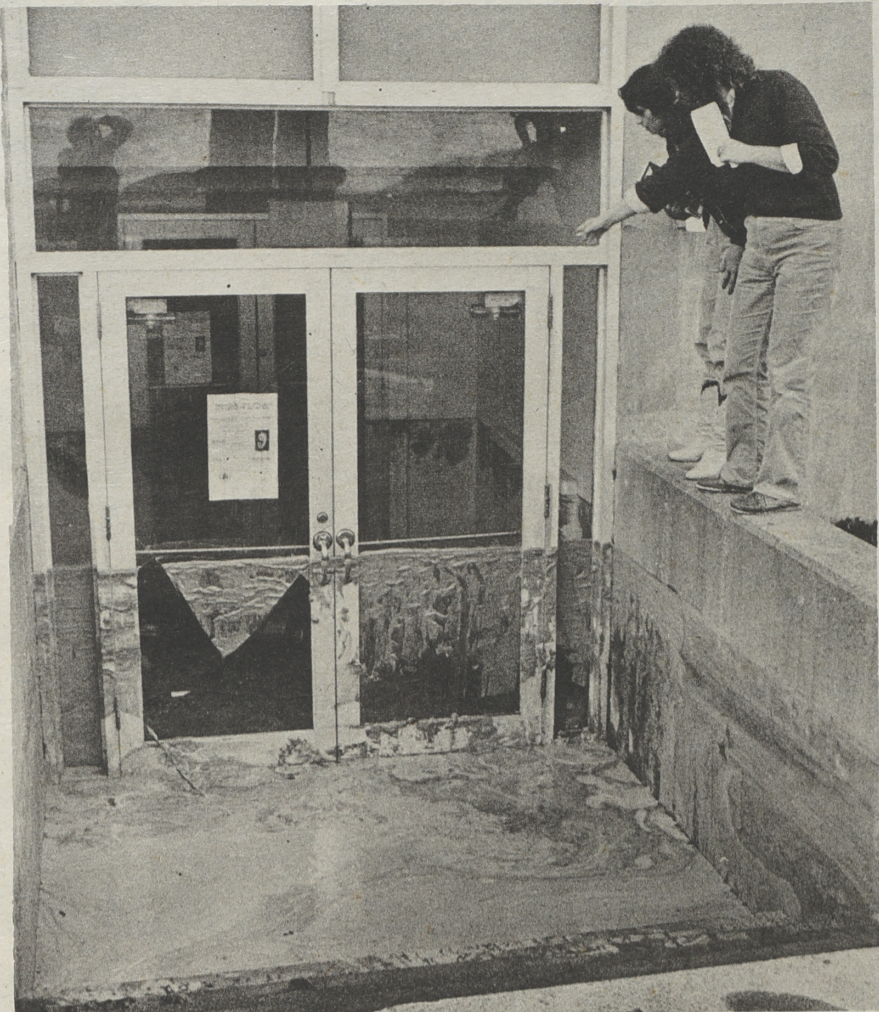
HIGH TIDE AT CRAIG LEE: Water gushed into the basement level of Craig Lee Hall after a water main broke nearby. Water rose to a level of over three feet before being turned off.
