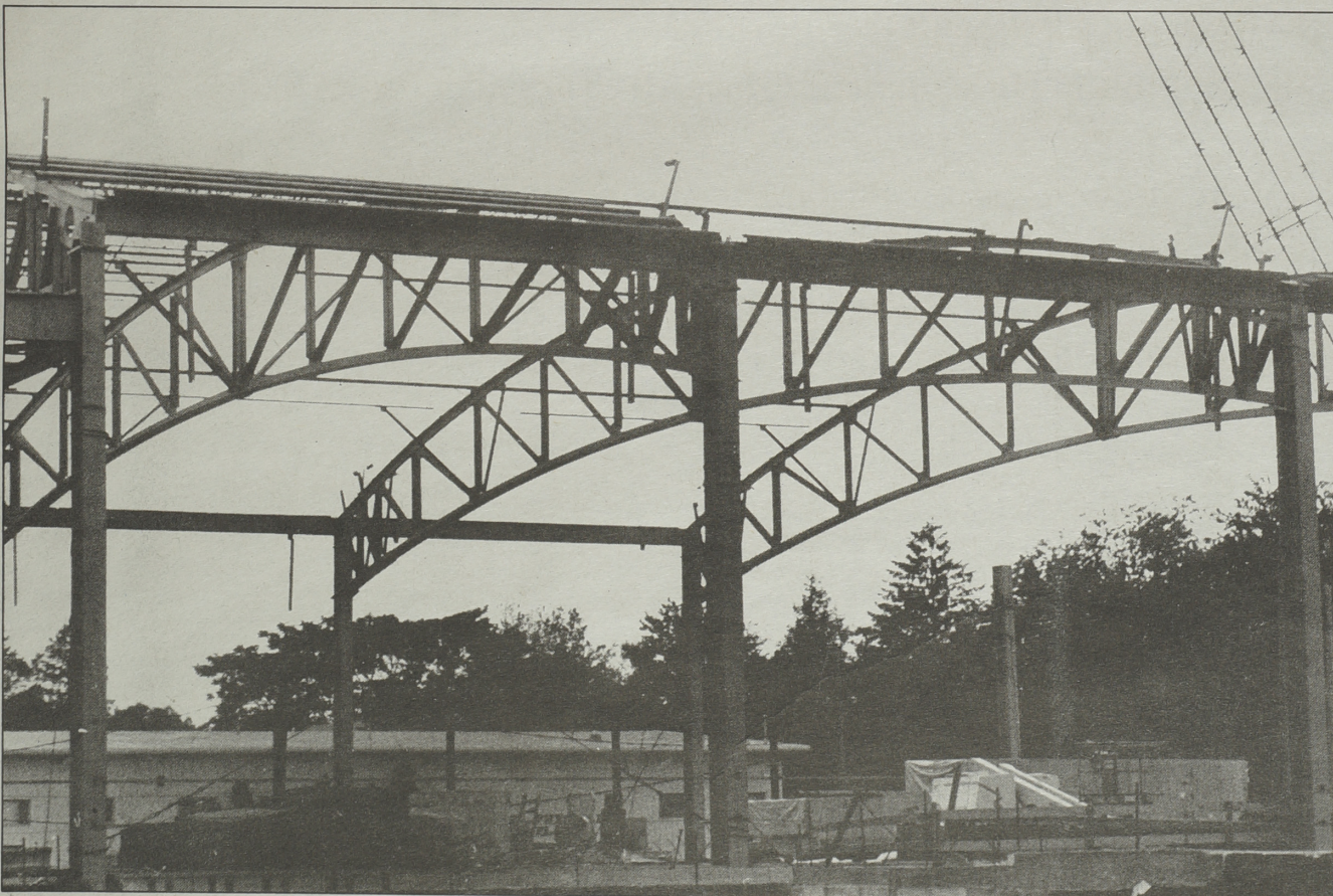
RAISING THE ROOF: The Health, Physical Education, and Athletic Complex is taking shape. The entire project is expected to be completed next year. What's News photo by Gordon E. Rowley.
