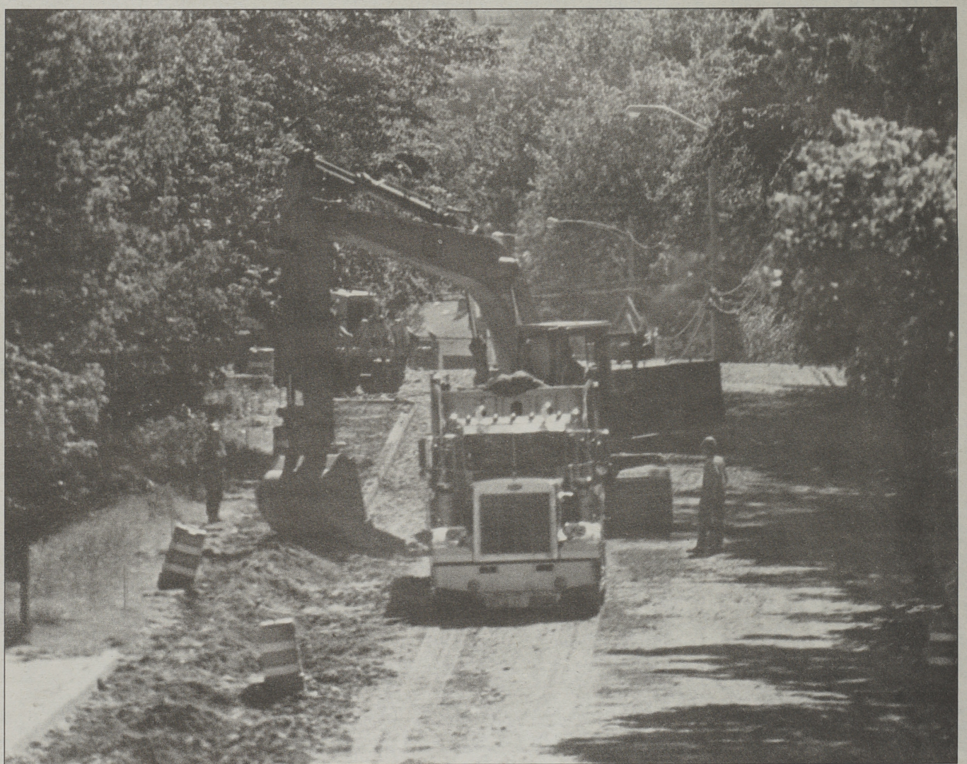
ON THE ROAD: The campus community and visitors will be pleased when the recently begun DOT road work is completed some time soon. In the meantime, patience, a "soft foot" and quiet anticipation of good things to come is the order of the day. Pictured above is College Road, the east entrance to the campus. The steep hill will be reduced by two feet when done. What's News photo by Gordon E. Rowley.
