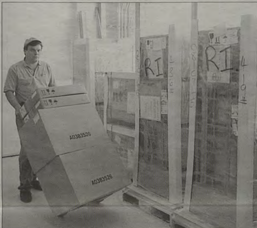
NEW TELEPHONE EQUIPMENT is moved into the second floor of Henry Barnard School by Guy Clermont, a technician with WILTEL, the company making the installation. The new system, valued at just under $1,000,000, is expected to be "up and running" by Oct. 1. (What's News Photo by Gordon E. Rowley)
